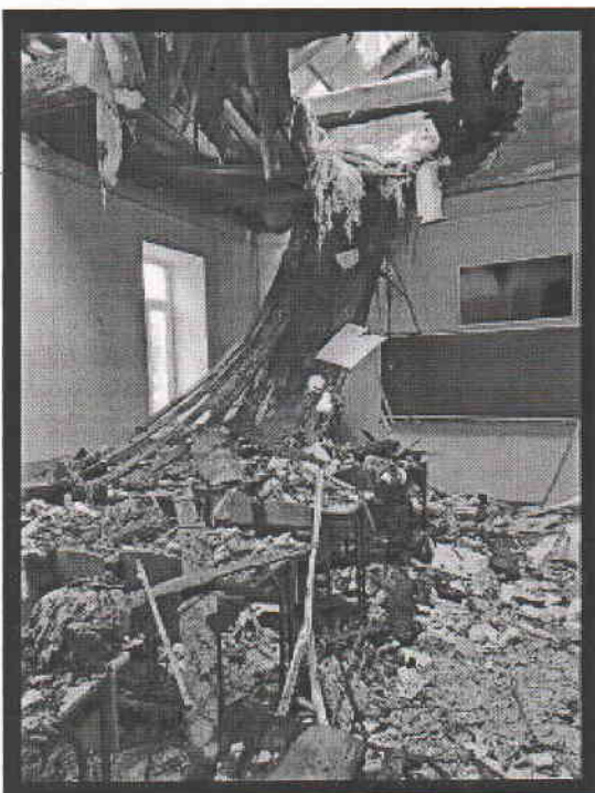
Scale of damage
